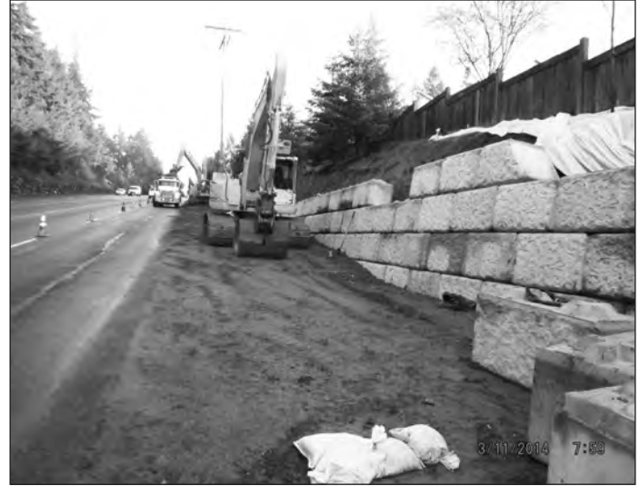
The Bridgeport Way West Phase 3B project is underway, and quickly moving along. Soon residents will be able to enjoy sidewalks through this section of our busiest street.
